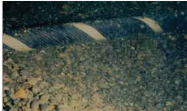
Figure 3.6: Image of a surface-laid cable taken during a post-lay inspection by an ROV. This image reveals the cable in the throes of burial by mobile gravel. Source: Transpower New Zealand and Seaworks.
