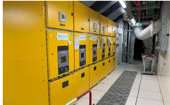
Electron Cyclotron Heating energization of the 22kV main switchgear
