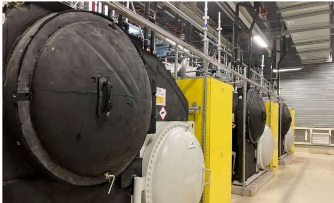
Chilled water system (condensers and evaporators)
