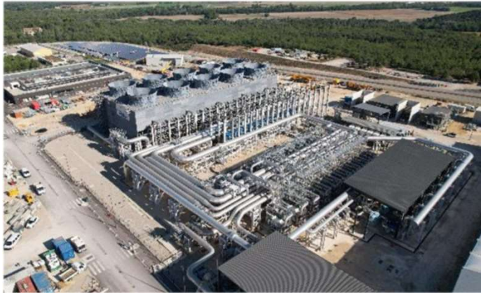
Heat rejection and cooling water system
